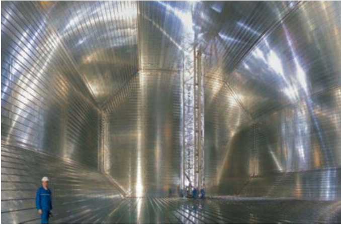
Photo: Yves Guillotin A 0.7 mm thick metal membrane of invar steel forms the first barrier in the tank; it is in direct contact with the liquefied natural gas at a temperature of -163 °C.
